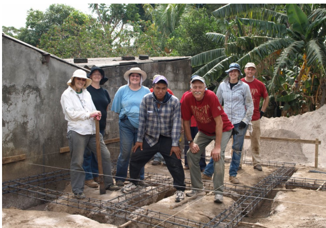
Board Member, Bruce Willis and his team working on a brick home in El Salvador in 2014.
